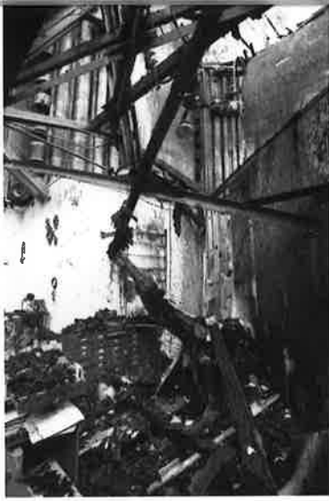
After fire-fighting crews left the site, the Cathedral's gift shop lay in ruins.
