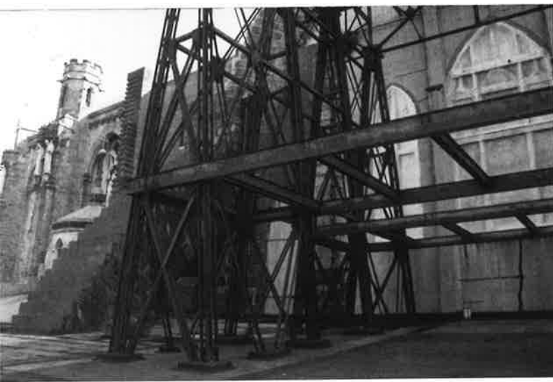
Construction during the 1930s left steel scaffolding on the roof of the North Transept.
